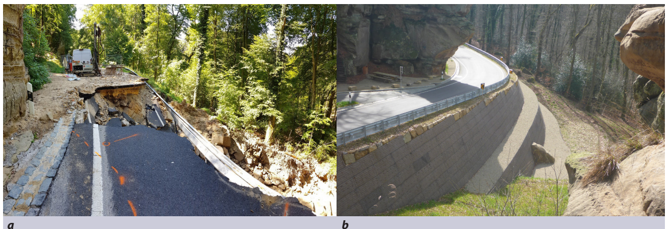
Figure 13: Situation before (a) and after (b) stabilisation.
